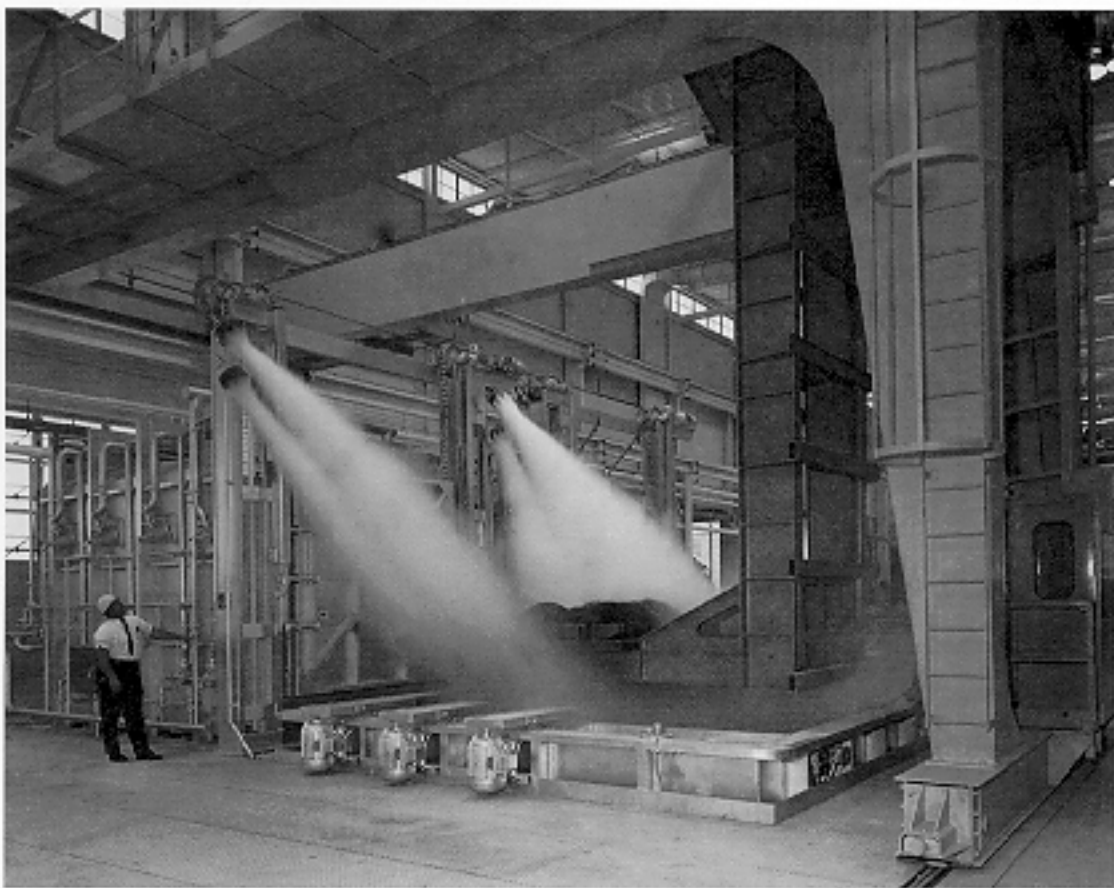
Start of CO 2 Discharge
